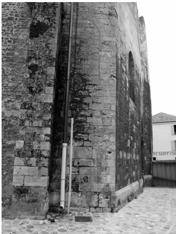
Figure 4. Notre-Dame d'Étampes, masonry break at the northwest corner of the chemin de ronde ; misalignment begins seven courses from ground level where it joins the north choir aisle. Photo by author.
