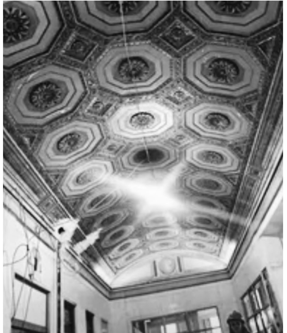
This original barrel vault ceiling will still be maintained with a modern style in the new lobby.
